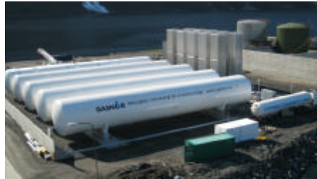
An existing terminal with similar tank configuration. Vertical structures at the back/right are evaporators to regasify the LNG. (Mosjøen, Norway)
